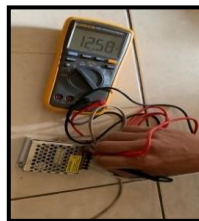
Gambar 5. Pengujian Power Supply
